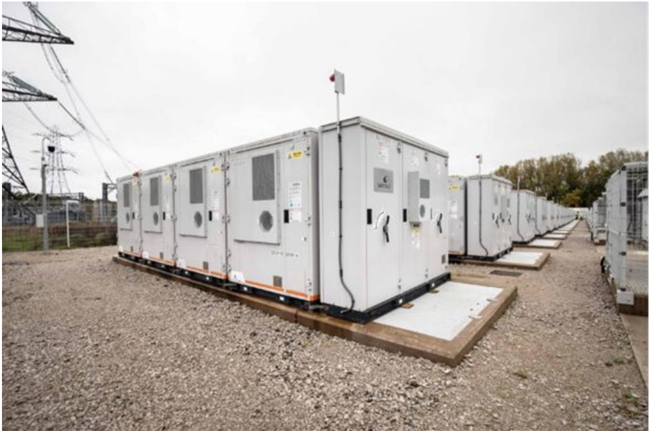
Plate 3.9: Example of an Operational BESS Compound
