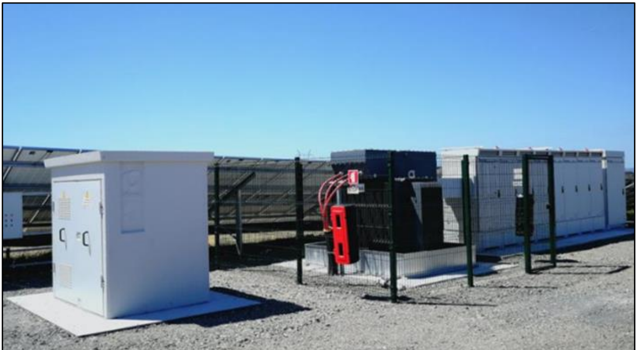
Plate 3.4 Typical Independent Outdoor Equipment (left to right: switchgear, transformer, central inverter)
